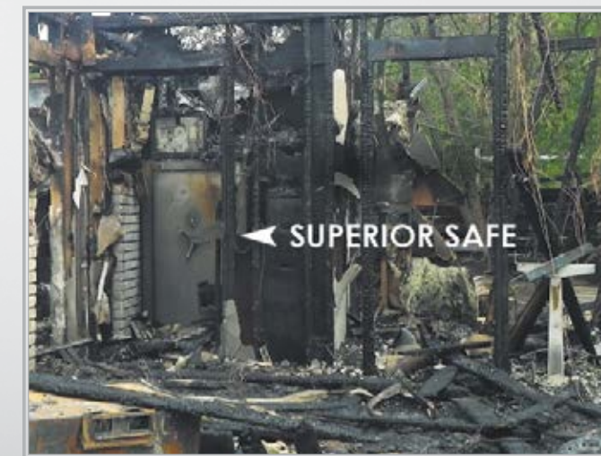
WHEN OPENED, THE CONTENTS WERE UNDAMAGED.
